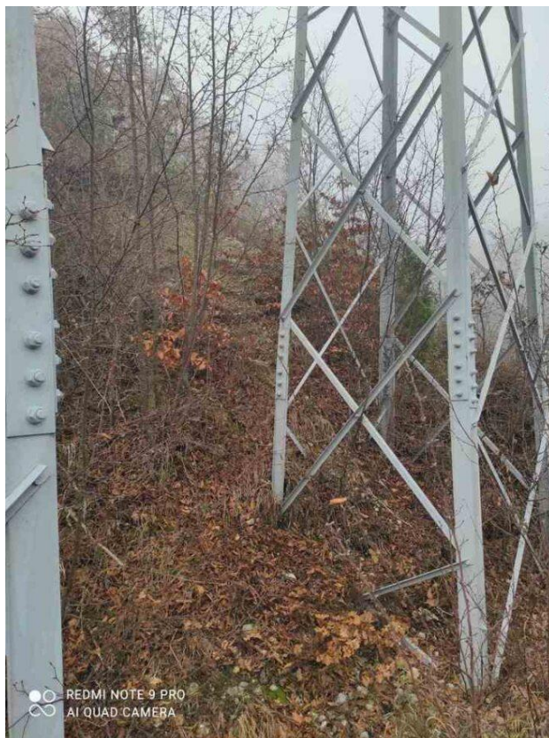
Sl. 7 DV 110 kV TS Sarajevo 1 – TS Sarajevo 10, portal SM 28A
