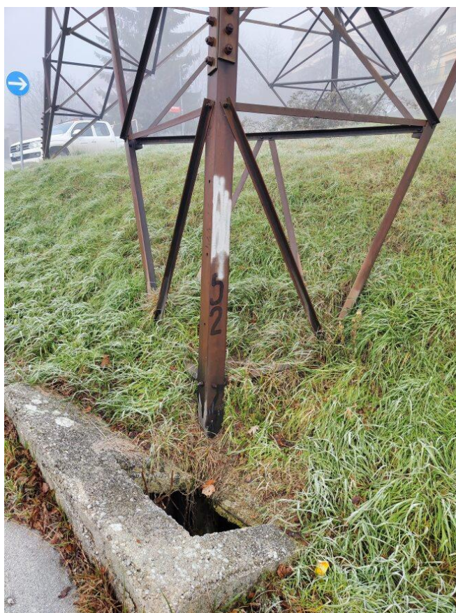
Sl. 4 DV 110 kV TS Sarajevo 10 – TS Sarajevo 5, SM 52 noga II
