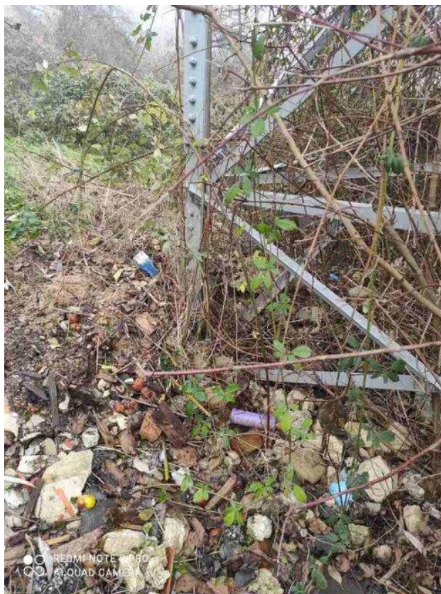
Sl. 9 DV 110 kV TS Sarajevo 1 – TS Sarajevo 10, SM 30 noga I
