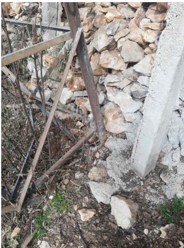
Sl. 3 DV 110 kV TS Sarajevo 10 – TS Sarajevo 5, SM 50 noga I
