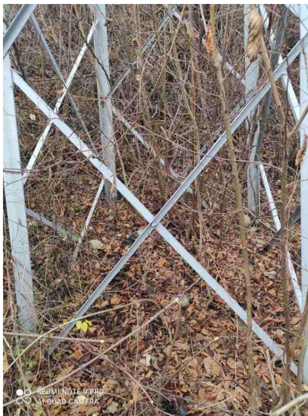
Sl. 8 DV 110 kV TS Sarajevo 1 – TS Sarajevo 10, portal SM 29
